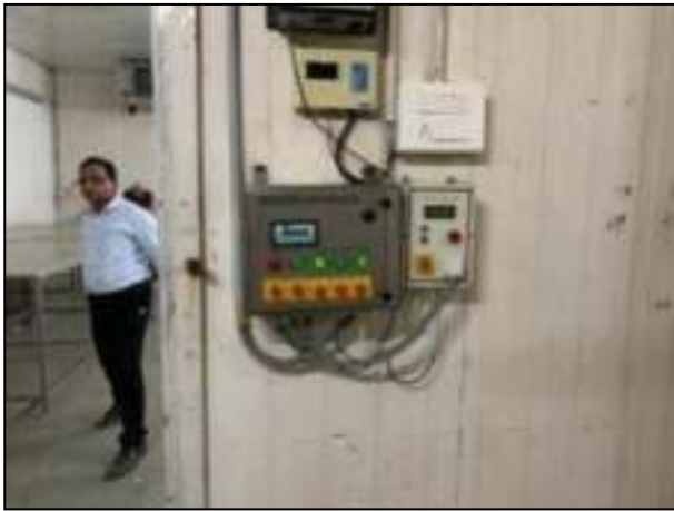
Ripening chamber controller, Export facility centre, Talegaon Dabhade
