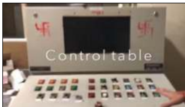
Control panel, Irradiation facility
