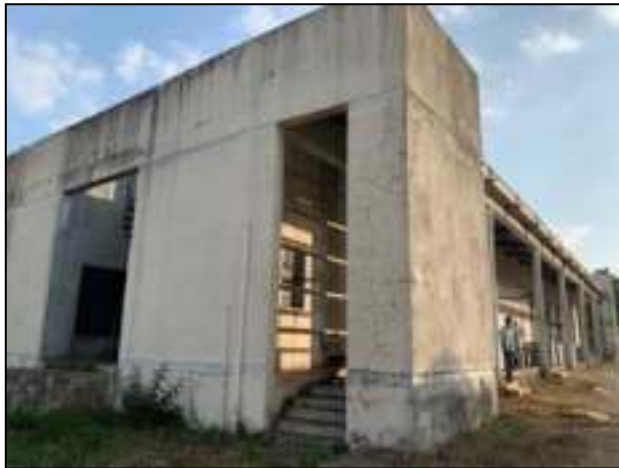
Export facility centre, Talegaon Dabhade
